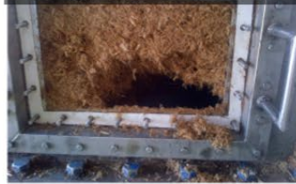
Bridging in drop chute
