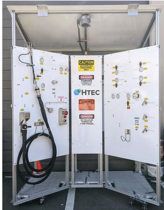
Figure 35 - HTEC GTM Control panel
