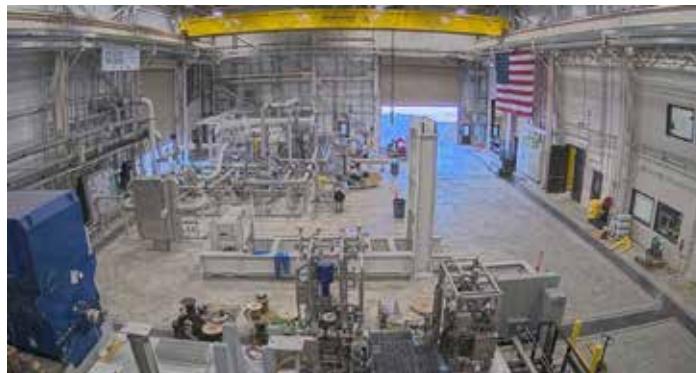
Assembly of supercritical carbon dioxide pilot showing welding of the piping network in progress in the facility
