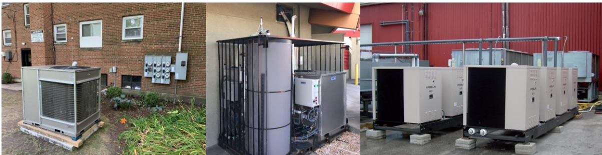
Figure 3: Commercial Installations of Sorption THP Equipment Including GTI Demonstrations of SMTI THPs in Multifamily Buildings (Left), Full-Service Restaurants (Center), and a Commercial Installation of Robur Equipment (Source: GTI/Robur)
