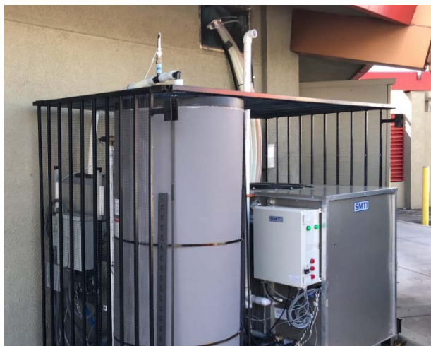
Figure 1: Commercial Gas Heat Pump Skid Package Installed at Host Site
