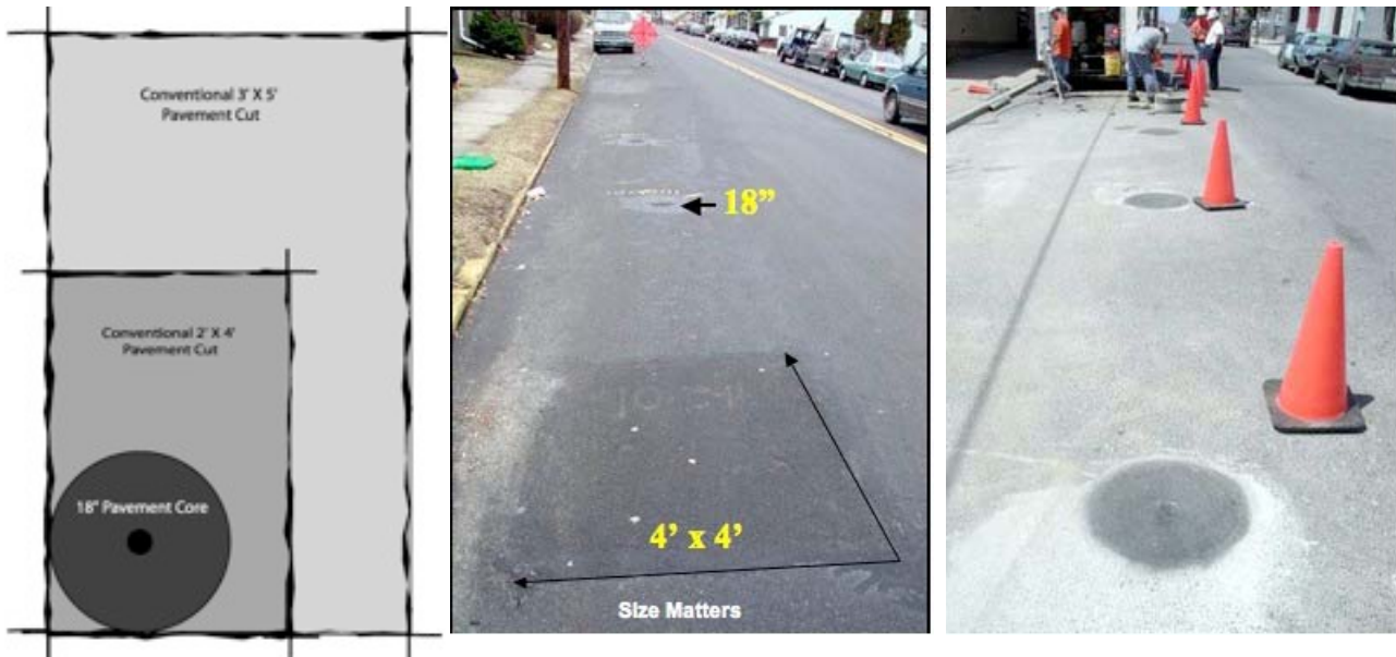
Figure 3: Size matters. (Left) An 18" diameter circular keyhole is less than half the size of a standard 2-foot x 4-foot cut and, because it is circular, has no corners in which to develop pressure cracks. (Center and Right) The large conventional repair of a 2-foot x 2-foot utility cut with a 1-foot cut back all around (making the area to be repaired 4-feet x 4-feet), is much more intrusive than the 18-inch keyhole behind or the series of keyholes on the right.
