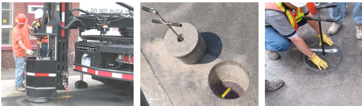
Figure 2: (Left) Rotary coring unit cores 18-inch diameter core; (Center) Core is removed and set aside. Vacuum excavation (not shown) is used to expose the infrastructure; (Right) After the work has been completed, the core is replaced and bonded back into the pavement as a permanent repair.
