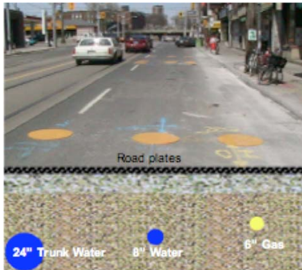
Figure 6: (View: Bathurst Street in Toronto looking north.) Pothole cores are cut to identify potential conflicts during HDD and temporarily capped with a circular road plate that allows traffic to flow uninterrupted on this busy thoroughfare while directional drilling takes place.
