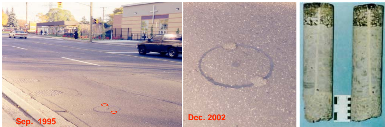
Figure 4: To test the effectiveness of the bond, Golder cut satellite core samples through the kerf of previously reinstated cores. These samples (right) showed perfect and complete bonding or adhesion of the Utilibond to both the surface of the core or coupon and the surface of the remaining pavement, as well as excellent “cohesion” through the joint itself. The light gray line, in the photograph, is Utilibond showing excellent bonding of the asphalt-concrete core (central area) to the undisturbed pavement (outer layer) with complete infilling of voids in pea gravel (bottom). The core which is directly in the wheel path of a transit lane of this arterial road showed no deflection from the time it was first reinstated in September 1995 (left) to December 2002 (center) notwithstanding the fact that during the seven year interval more than 145,000 transit buses and 13 million commercial and other vehicles have passed directly over the keyhole with no apparent weakening or other degradation of the reinstated core or the adjacent road system or paved surface.
