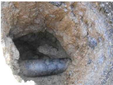
Exposed 6" steel water pipe
