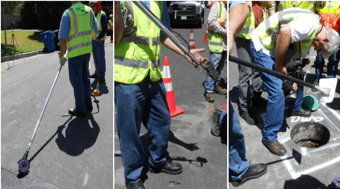
Long-handled tools used to grind away the pipe coating, cadweld the wire to the pipe, and re-coat the pipe and exposed wire
