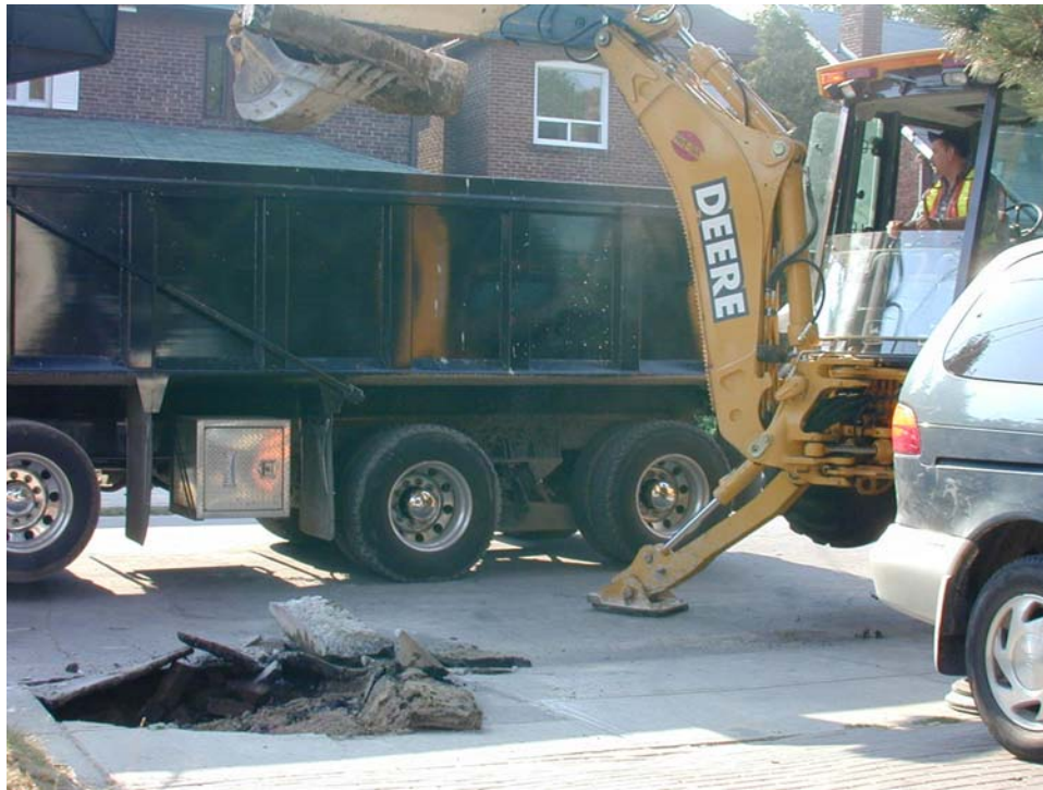
Photo 1 – Traditional utility service cut.
