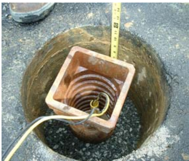
Install test station level with pavement and backfill around box with 3-4 inches of pea gravel.
