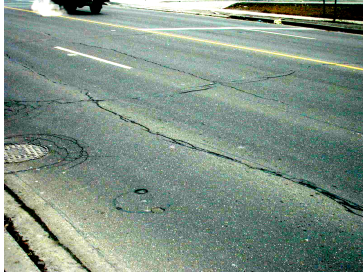
Figure 5. Pavement core reinstated in bus lane with Utilibond in 1995 still in perfect condition seven years later in 2002.
