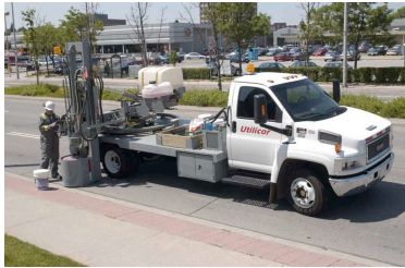
Figure 1. The Utilicor coring unit operates through a complete 270° arc, allowing the truck to be positioned on the shoulder or off the traveled surface to minimize traffic disruption.
