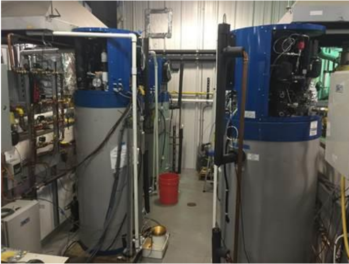
Figure 4: 3 rd Generation Prototypes Undergoing Reliability Testing at GTI
